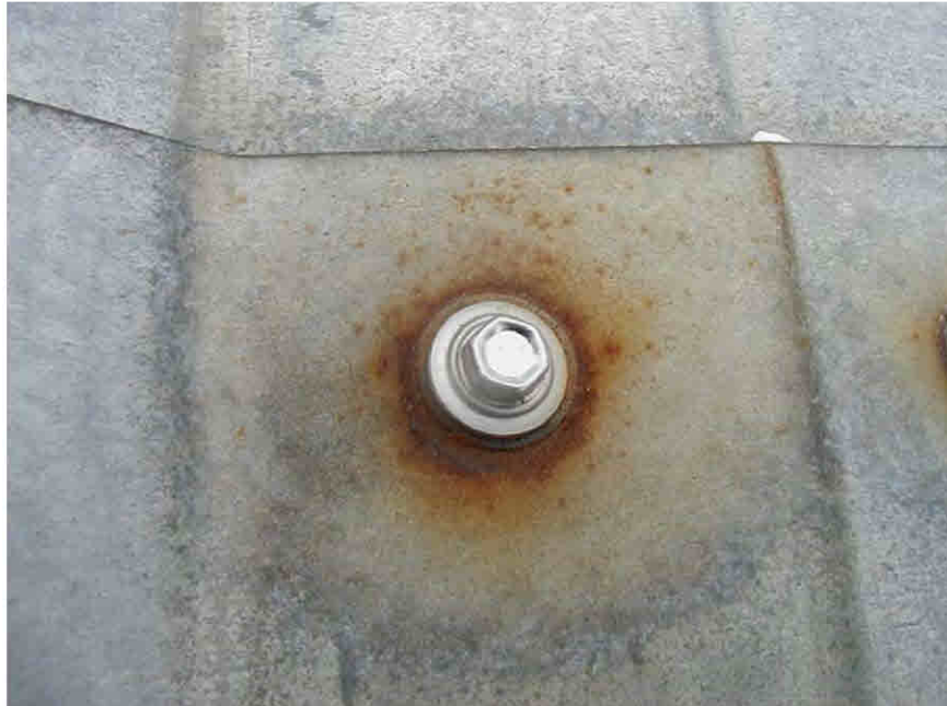
Figure 27. Photograph of red rusted metal filings on the surface of bare GALVALUME® roof panel around a screw.
