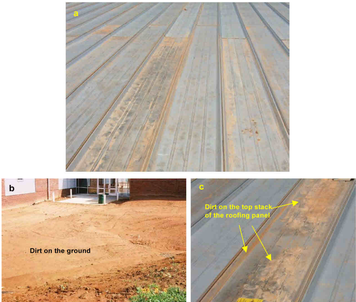
Figure 1. Photographs of stains and inconsistent appearance of a bare GALVALUME ® roof (a), dirt on the ground at a building site (b), and dirt concentrated on the roofing panels on the top of the stack (c).
