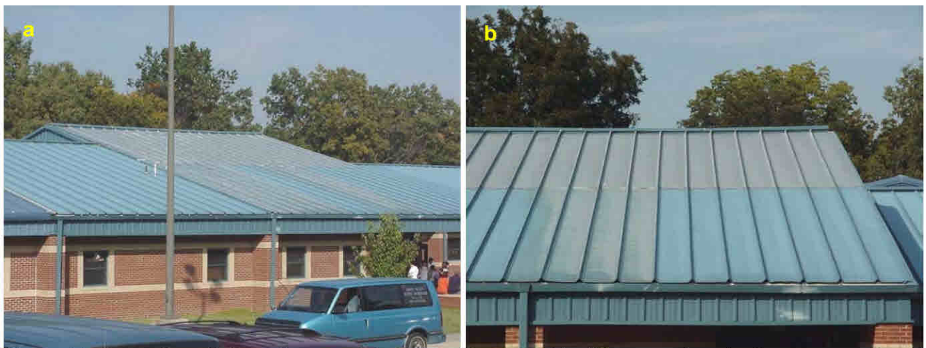
Figure 44. Non-uniform fading of a prepainted roof with noticeable differences in color from one section to another section (a) and its close look (b).
