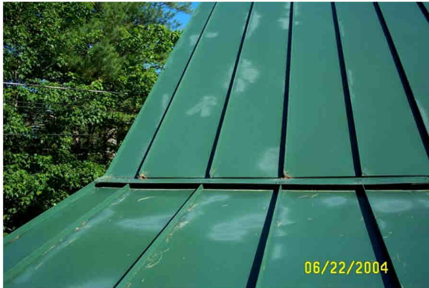
Figure 45. Differential chalking and fading appearance on the prepainted GALVALUME® steel roof with improper touch-up paint.
