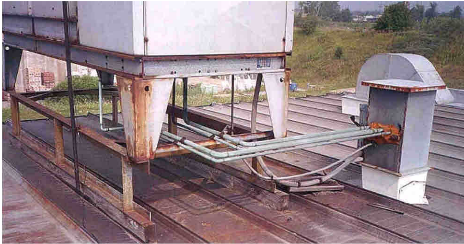
Figure 36. GALVALUME ® roof panel corrosion due to condensation water runoff from the copper pipes.
