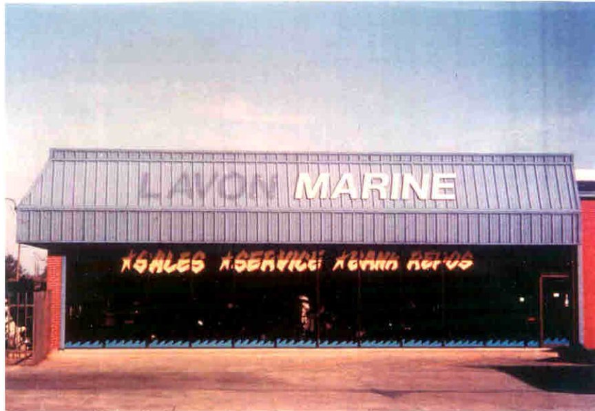
Figure 43. Color fading of the paint on prepainted panels due to UV light from the sun.
