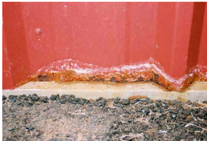
Figure 18. Premature corrosion at the bottom edges of the prepainted GALVALUME® panel caused by direct contact with the concrete foundation.
