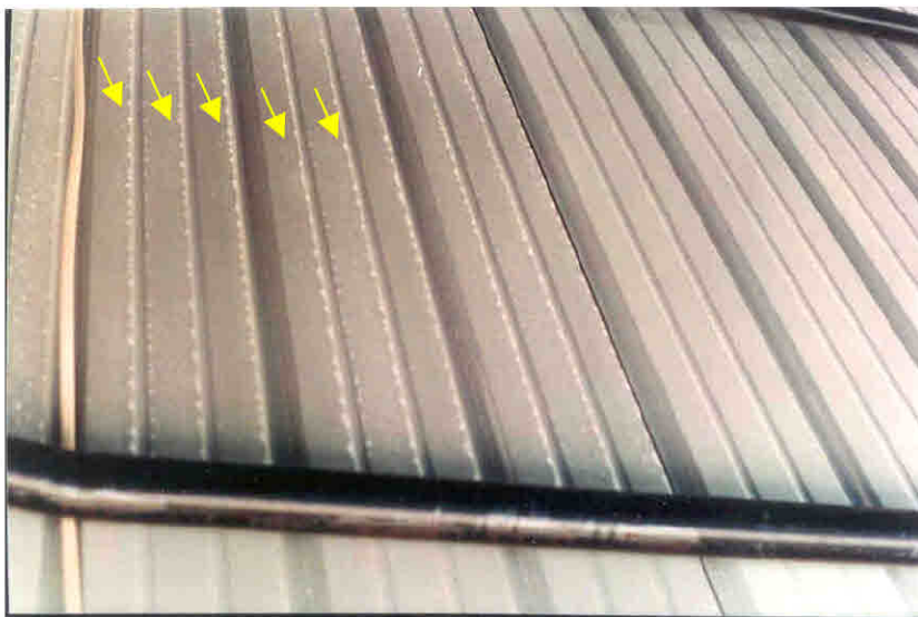
Figure 42. Photograph of the backside of the roofing panel shows condensation accumulating along the ribs of the panel as the arrows indicate.
