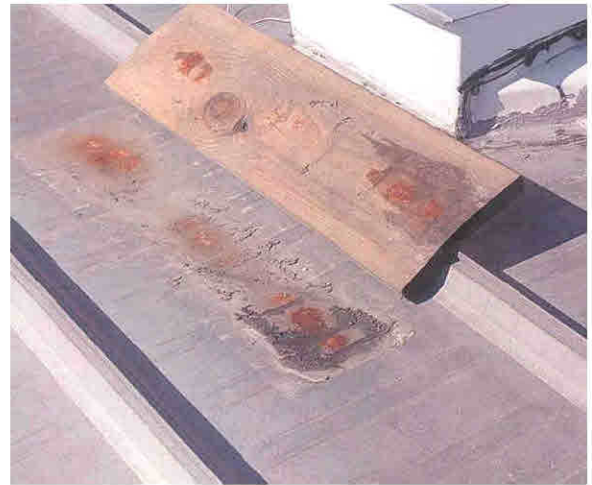
Figure 31. Corrosion occurred under the treated lumber because chemicals, particularly copper compounds, leached from the wood accelerating the corrosion.
