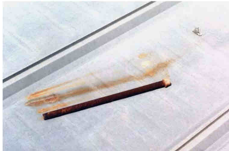
Figure 32. A piece of metal tube left on the roof caused staining and corrosion of the roof panel.
