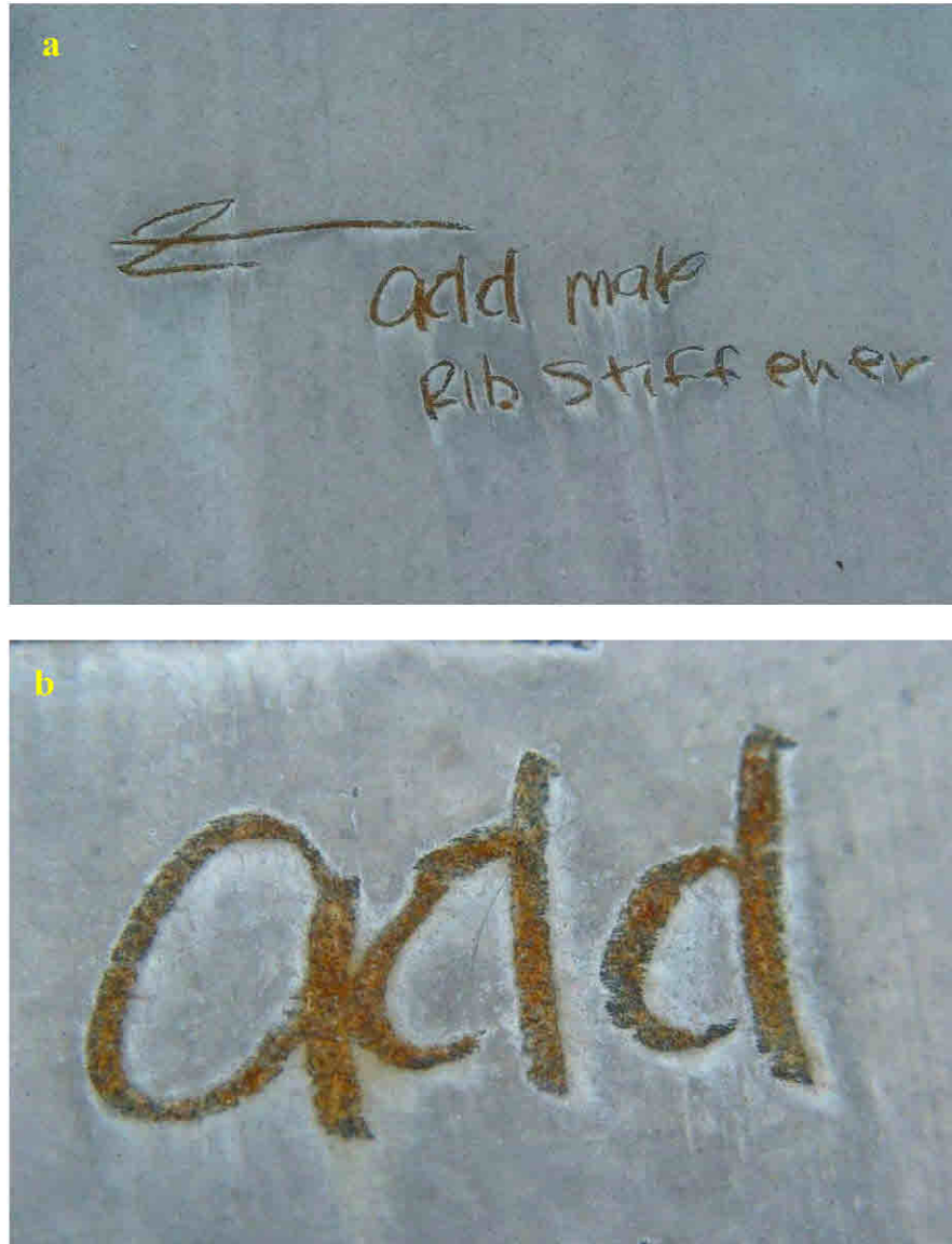
Figure 29. Photographs of pencil mark corrosion on galvanized steel sheet (a), and a magnified view of the mark (b).
