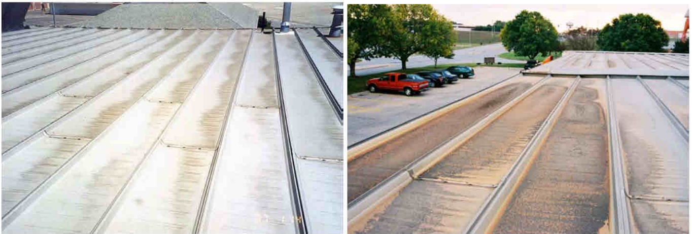
Figure 22. Photographs of water ponding on a GALVALUME® roofs due to improper slope of the roof.
