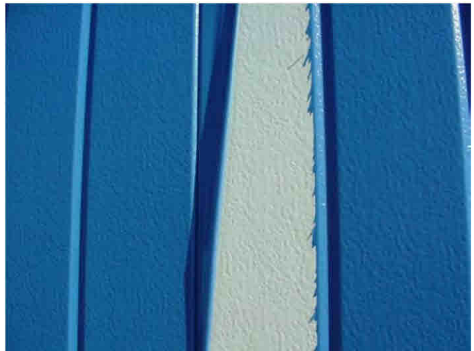
Figure 49. The primer remained on the panel where the topcoat peeled off.
