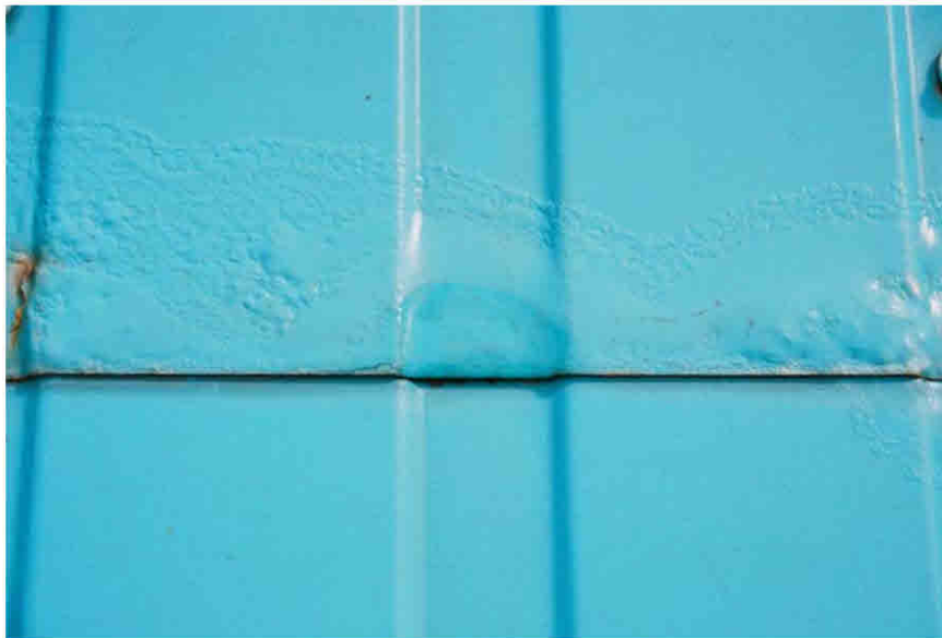
Figure 25. Paint blistering on a prepainted GALVALUME® roof caused by poor end lap sealing.
