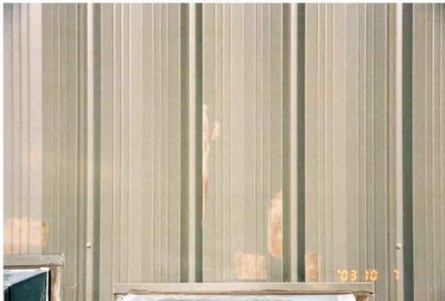
Figure 46. Differential chalking and fading appearance on prepainted hot-dip galvanized steel siding with improper touch-up paint.
