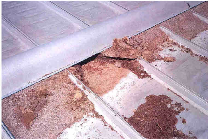
Figure 30. The wood chip debris piled near the ridge cap caused heavy corrosion of the roof panel due to water being retained by the debris.
