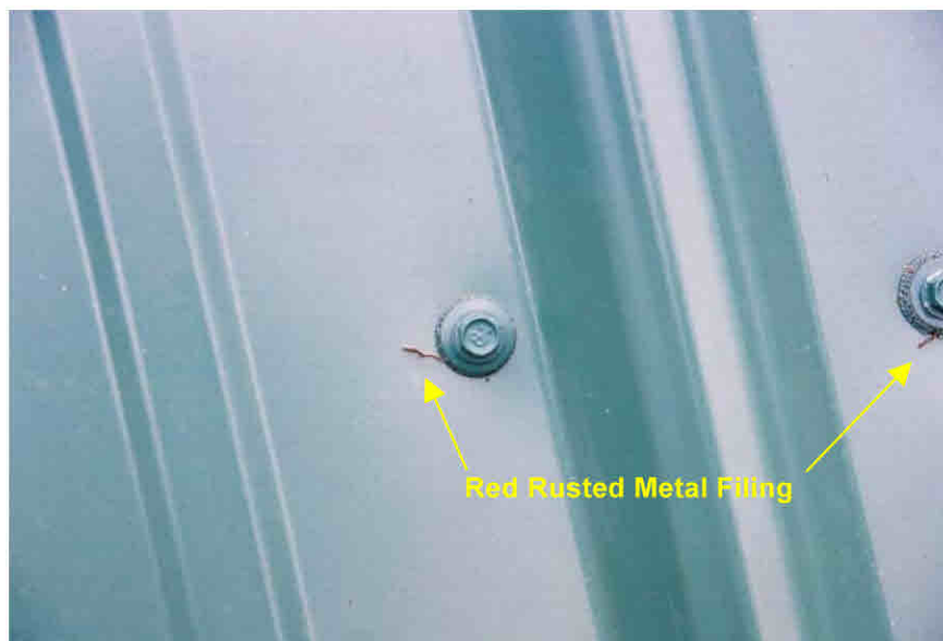
Figure 28. Photograph of red rusted metal filings from the screws on a prepainted GALVALUME® roof panel.
