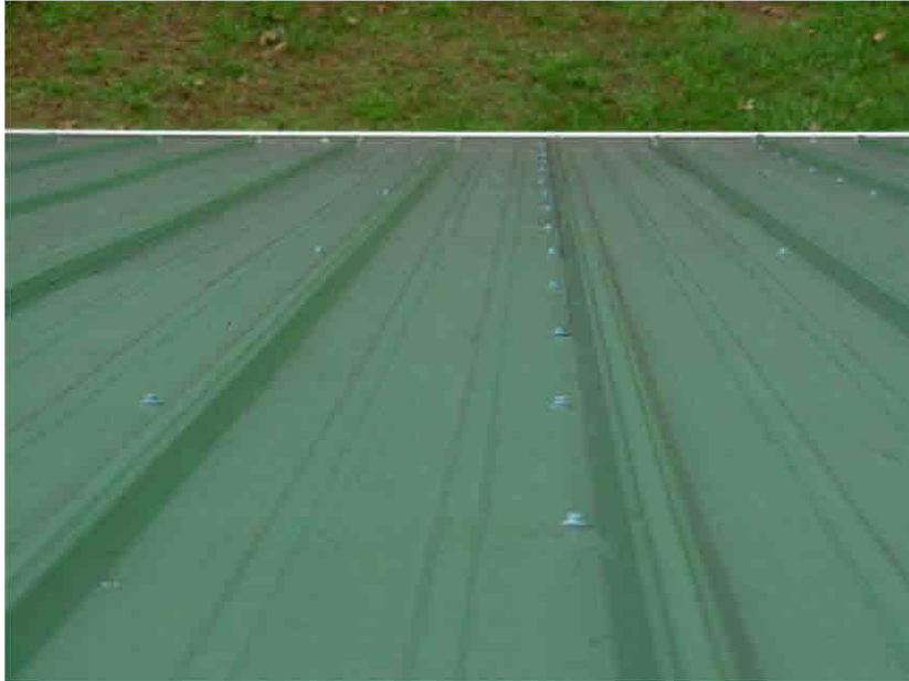
Figure 13. Photograph of the prepainted galvanized steel roof with non-matching screws.
