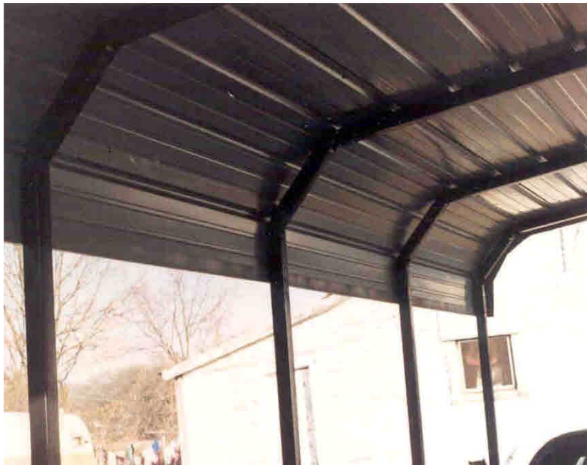
Figure 41. Improper roof profile design of a pole building with open sides does not allow rainwater to runoff along the curvature of the roof.
