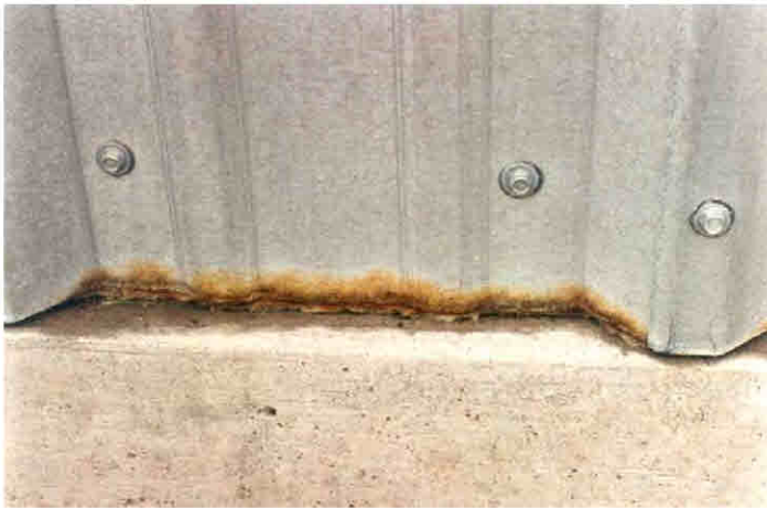
Figure 16. Premature corrosion at the bottom edges of the GALVALUME® panel caused by insulation wicking.
