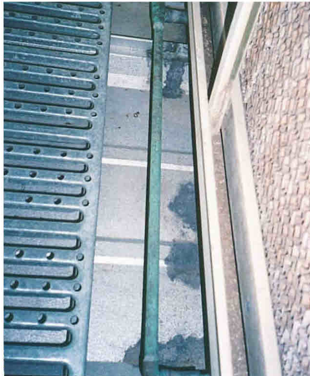
Figure 37. GALVALUME ® panel corrosion due to condensation water runoff from the copper pipes.
