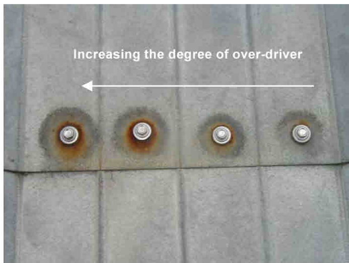
Figure 11. Photograph of the over-driven fasteners. The corroded area around the fastener increased with increasing depth of depression.
