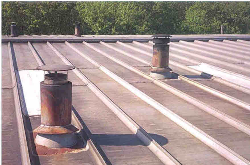
Figure 35. The GALVALUME® roof was corroded around the roof stacks.
