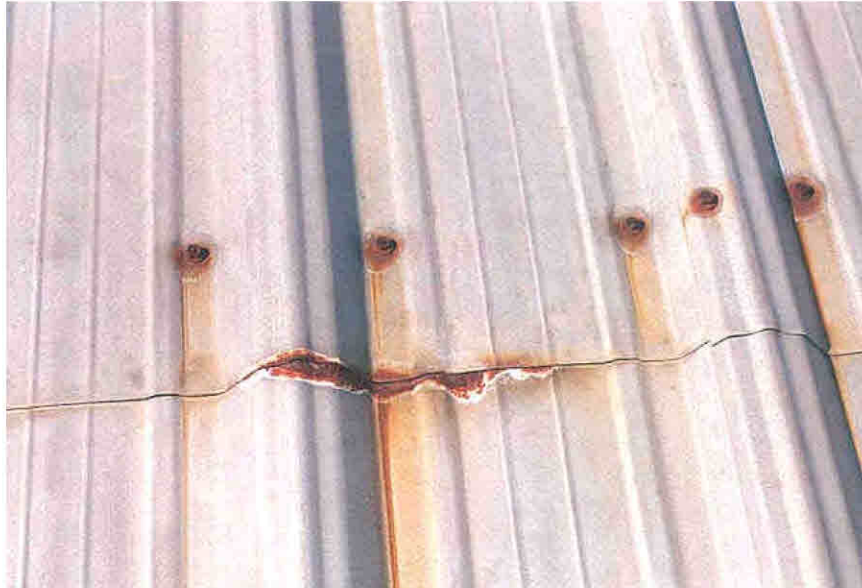
Figure 24. Crevice corrosion caused by poor end lap sealing on a GALVALUME® roof.
